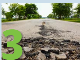
3 Poorly Maintained Roads
