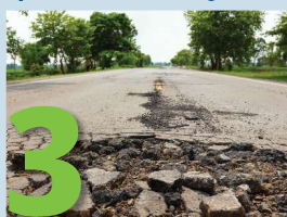
3 Poorly Maintained Roads
