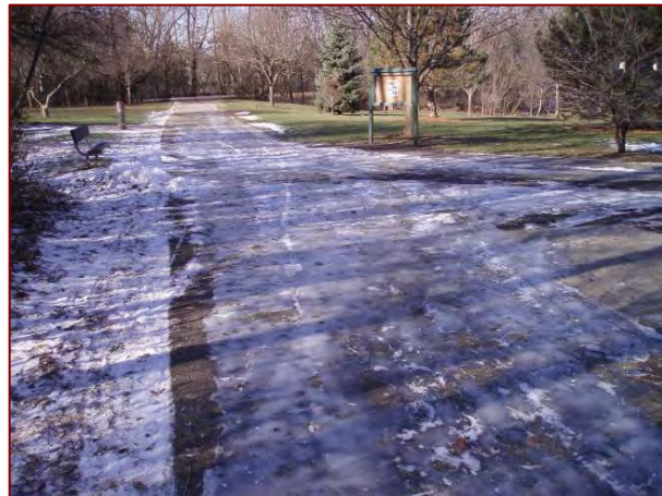
Figure 24. Snow and ice accumulation on the Constitution Trail creates hazardous walking and bicycling conditions
