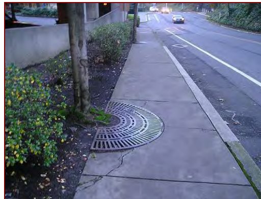
Tree well grates should be flush with the sidewalk surface
