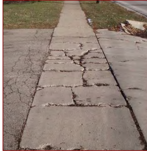
Figure 25. Damaged sidewalk on Willow Street's north side east of Main Street
